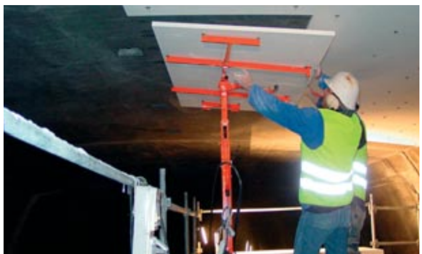
Below: Calcium silicate boards being fixed to a tunnel soffit. Picture by kind permission of ASFP member - Promat UK Ltd
